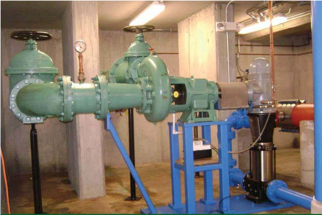
The Torrington Water Company's Hydropump, installed and operating. Note the custom made mounting assembly designed by AVI International in Torrington.
