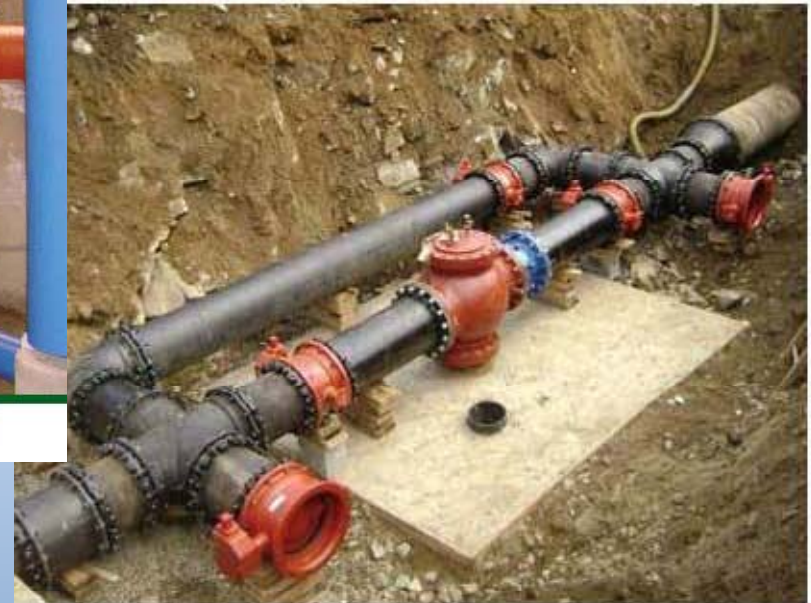
Construction of the bypass pipes needed to direct raw water to the basement of the pumping station. Virtually all of the installation was accomplished by Torrington Water Company employees.
