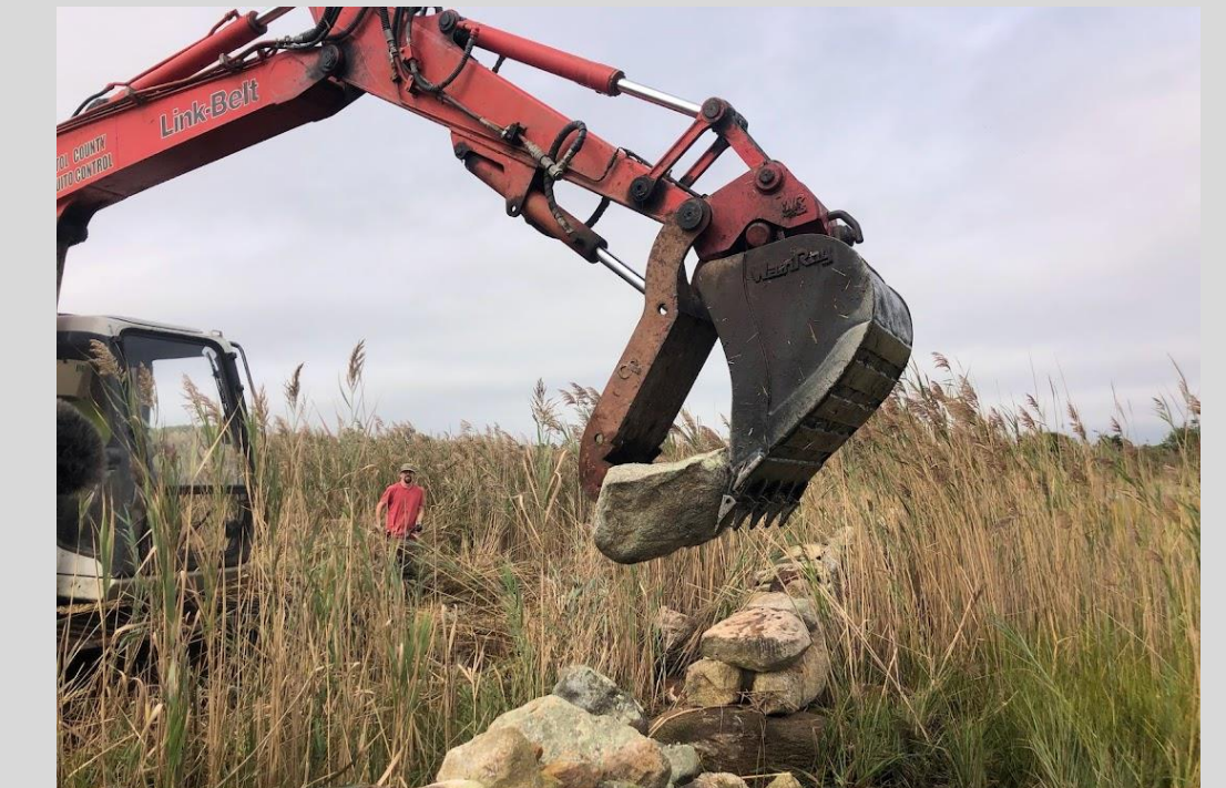
Bristol County Mosquito Control Project's low ground pressure excavator removing sections of stone wall to drain impounded water in marsh migration corridor
