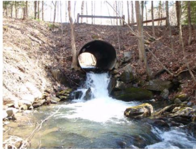
Figure 20. Perched culvert beneath Ryan Road.
