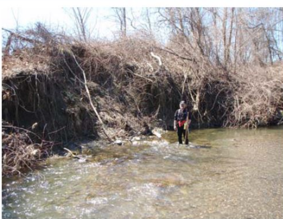
Figure 14. Mass failure in lower M01-B
