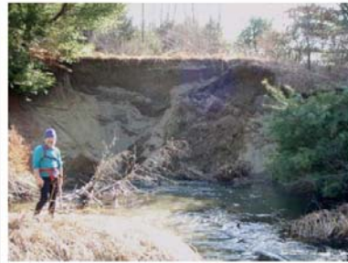
Figure 17. Large mass failure in upper M02
