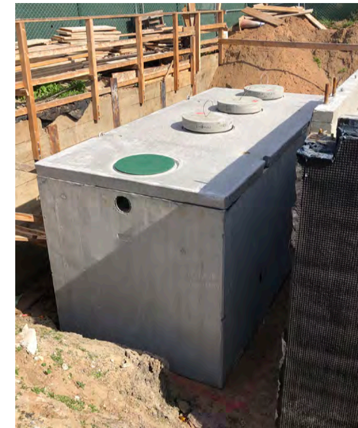
6,000 GALLON UNDERGROUND CONCRETE WATER STORAGE TANK
